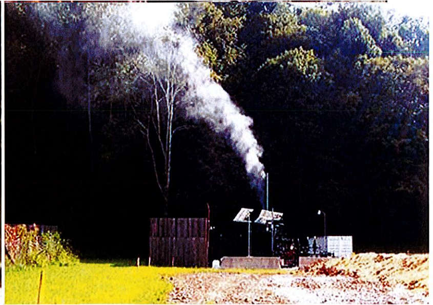
Condensate/Brine Tank On Pad
